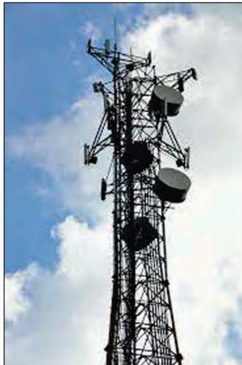
Figure 5: A microwave tower
