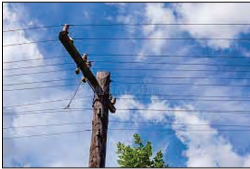
Figure 1: Wooden telegraph pole with open wire
